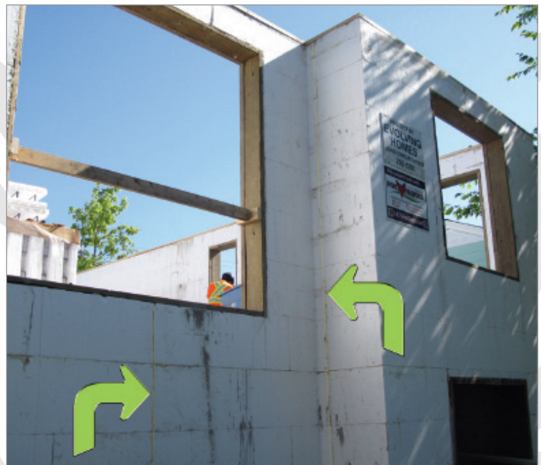
Here is a job, post concrete, that has been constructed exactly to the building dimension by properly stacking seams.
